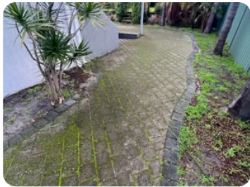
04 Paths & hardstand Slip risk on shaded paving and entries.
